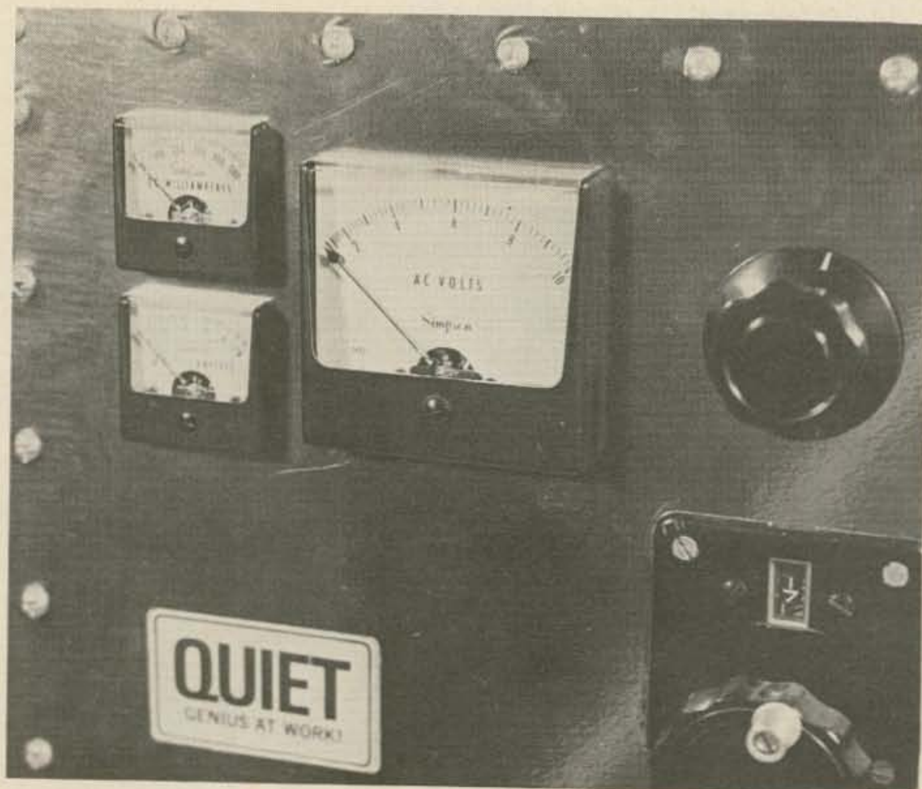
Detail of panel meters.
