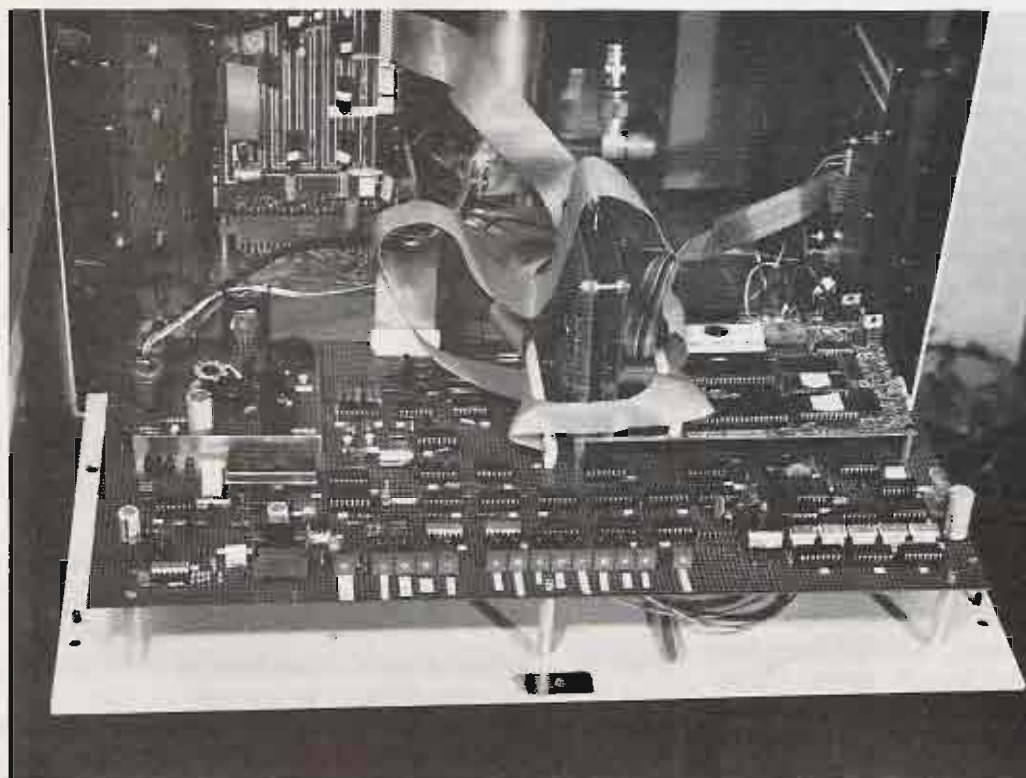
Photo C. Repeater control board. Main board mounts on the cabinet's "front door" Clockwise from upper right are CPU-1A microcomputer, audio delay line, audio mixers, phone patch, and dc-dc converter.
