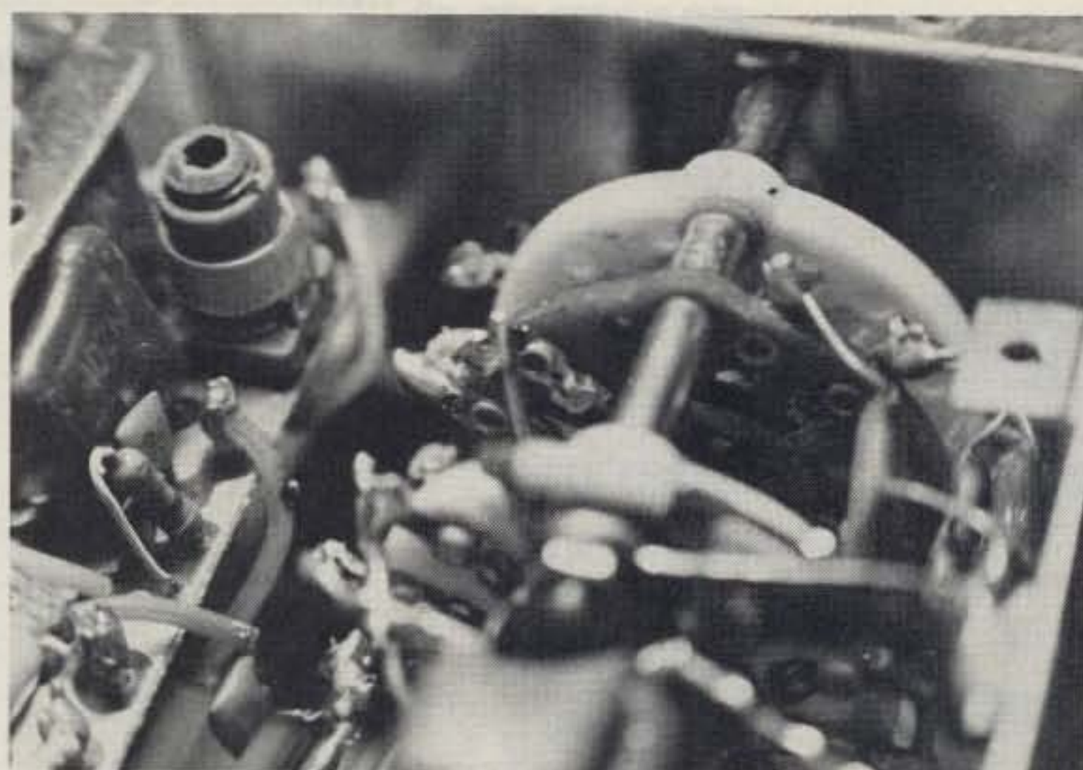
Photo C. Wafers j, k, l, and m are shown in this photo. Note the added tab in the center of the photo on S1l, held in place by the rivet and Super Glue.
