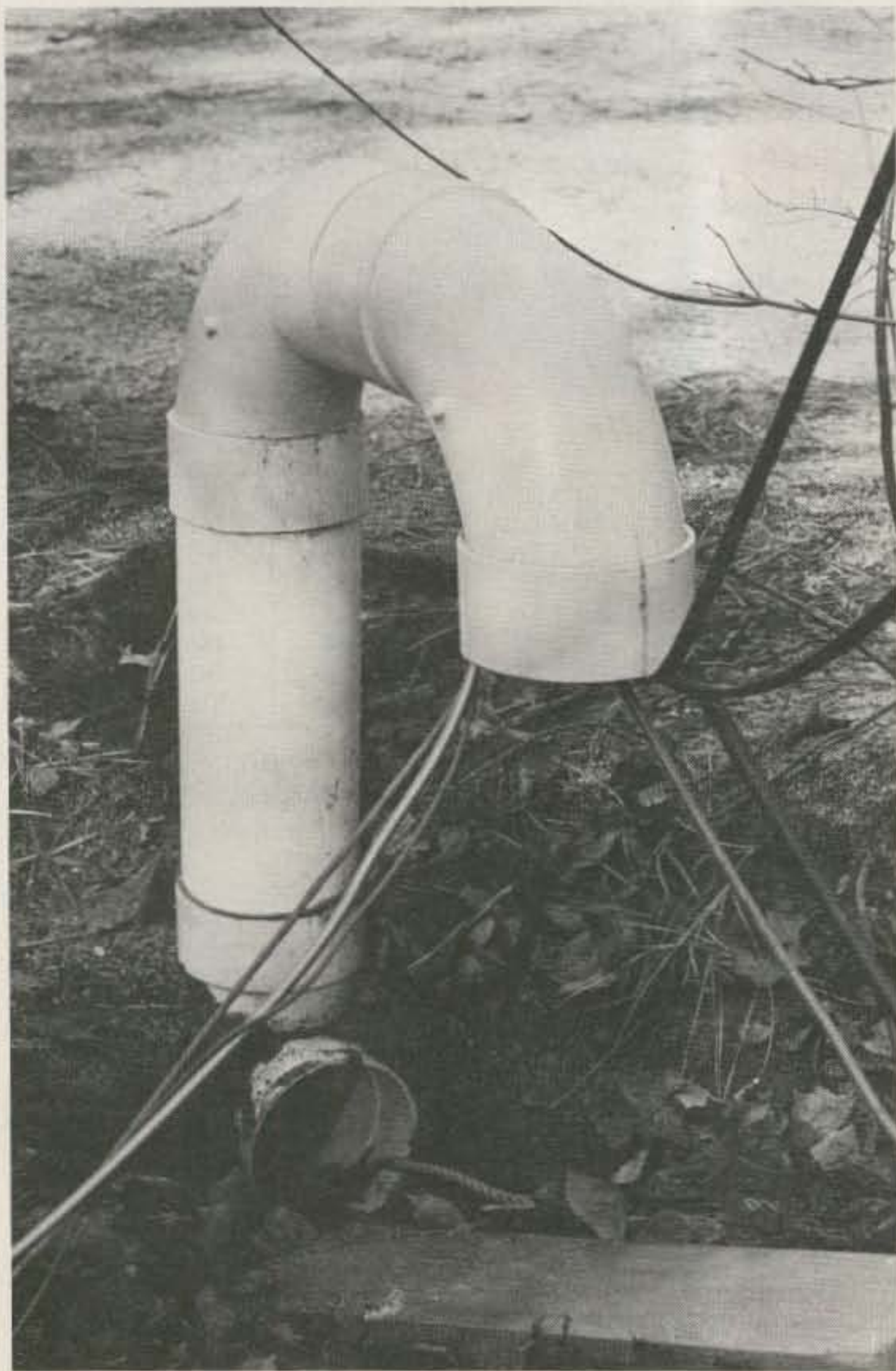
Photo A. The PVC pipe has a couple of elbows on the end of it to keep out rain and snow. A pull rope is left in the pipe to move additional antenna and rotor cables through; otherwise, the open end is capped and covered with dirt.
