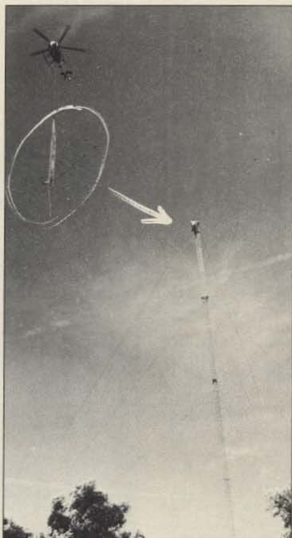
This tower, taller than the Statue of Liberty, required a helicopter to lift the top 21-foot section into place.
