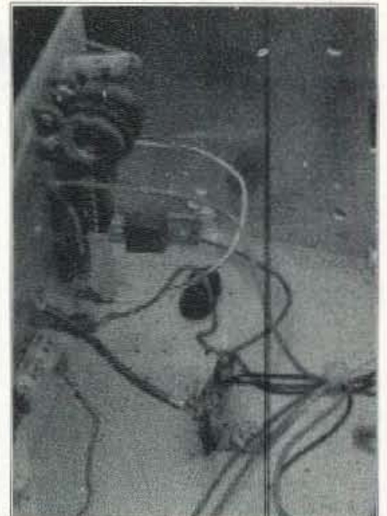
Photo B. Notice the burnt insulation near the terminal strip. The two trimmers on the top of the PC board set the voltage and current trip points for the supply.
