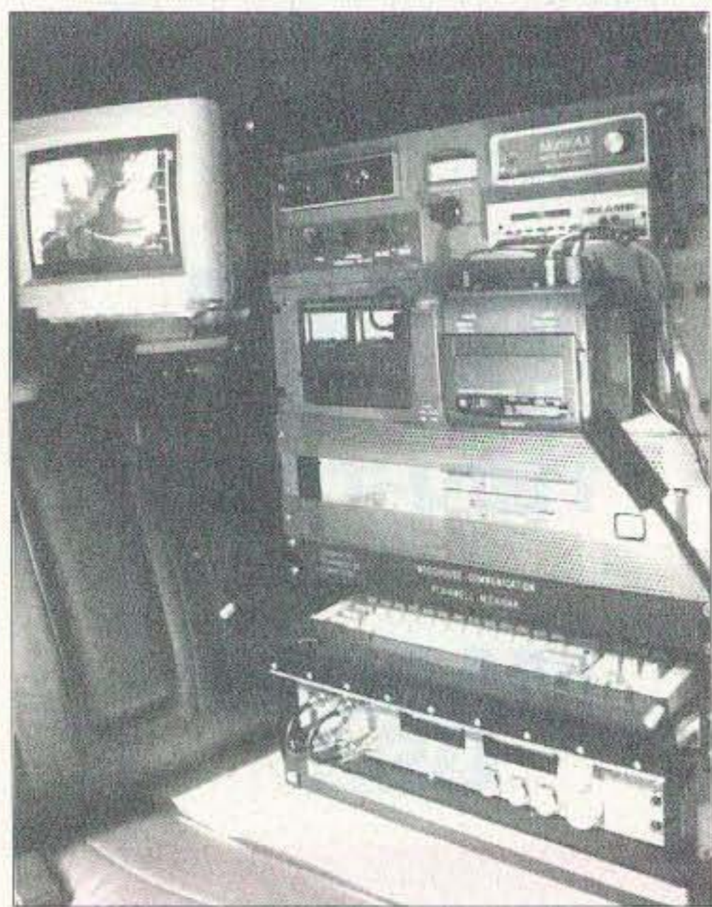
Photo B. Inside view of the operating position in the back seat. Note power monitor control panel at bottom, keyboard drawer for storage while in motion, and printer on top of rack.
