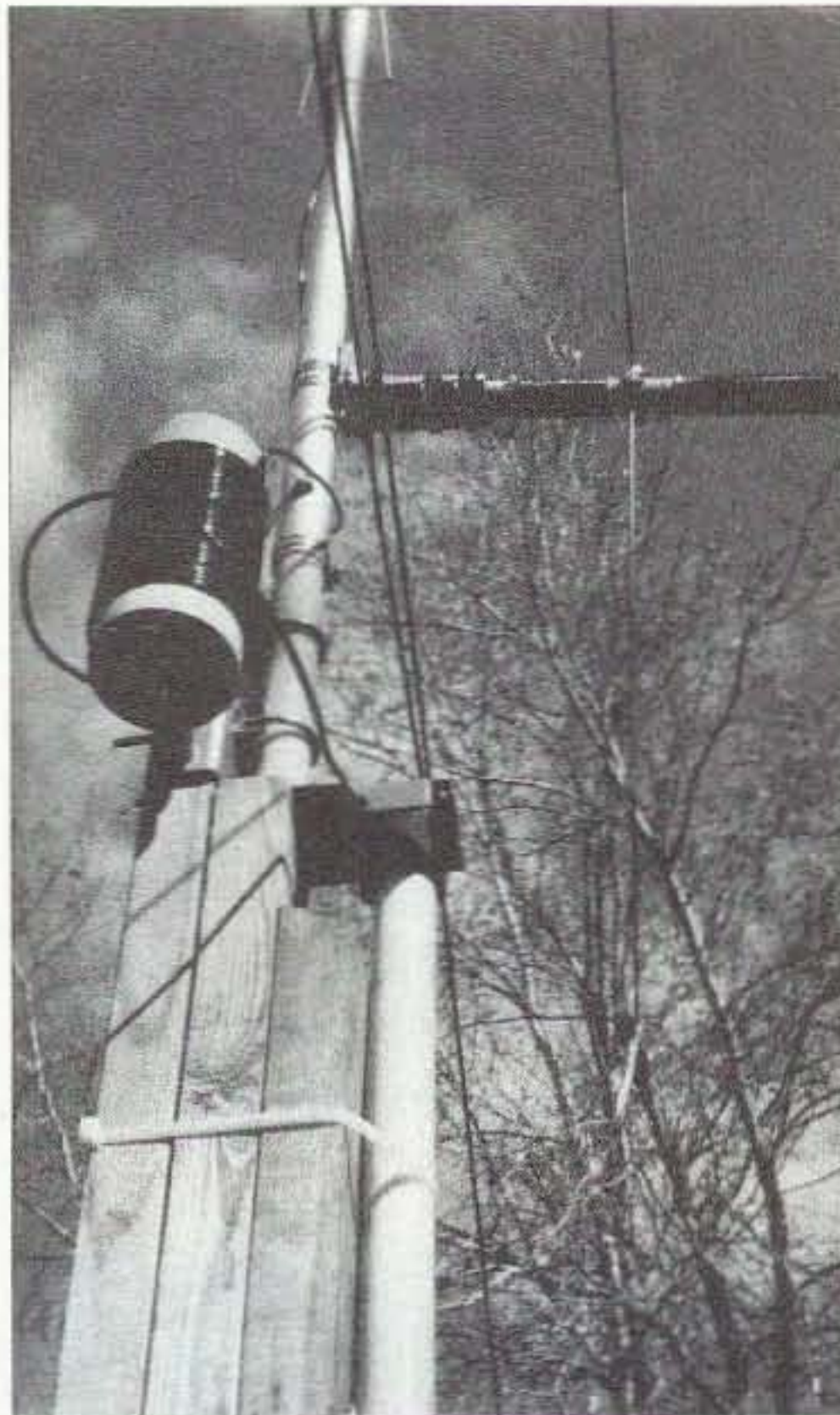
Photo G. Base of antenna showing balun and loading coil assembly.
