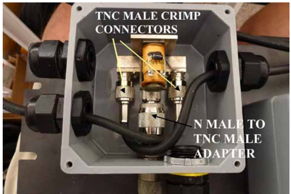
Figure 6: Antenna Coax Relay mounted in a weatherproof plastic electrical box. Relay has TNC connectors and is powered by 28VDC. Compression fittings are used to prevent water from entering the box. Separate boxes are used for the VHF and the UHF elements so all combinations of linear polarity are available (H-H, V-V, H-V and V-H).
