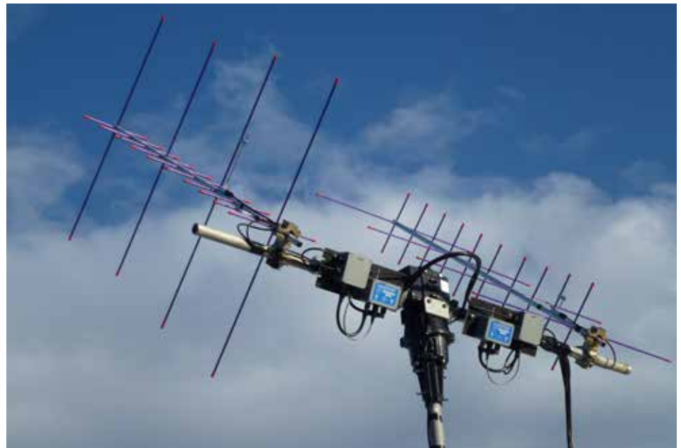
Figure 2: Showing the Extended Arrow antennas along with preamps and coax relay boxes.
