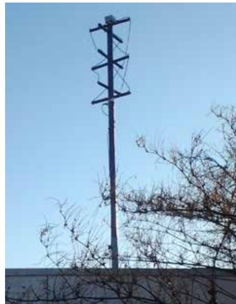
Figure 2. Monitoring station antenna
