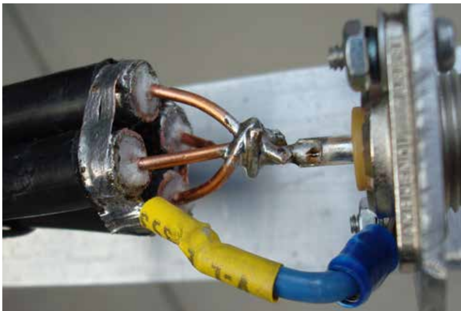
Figure 4 — Shields of the four RG-11/U matching sections are bonded together and connected to ground by a short lead.
