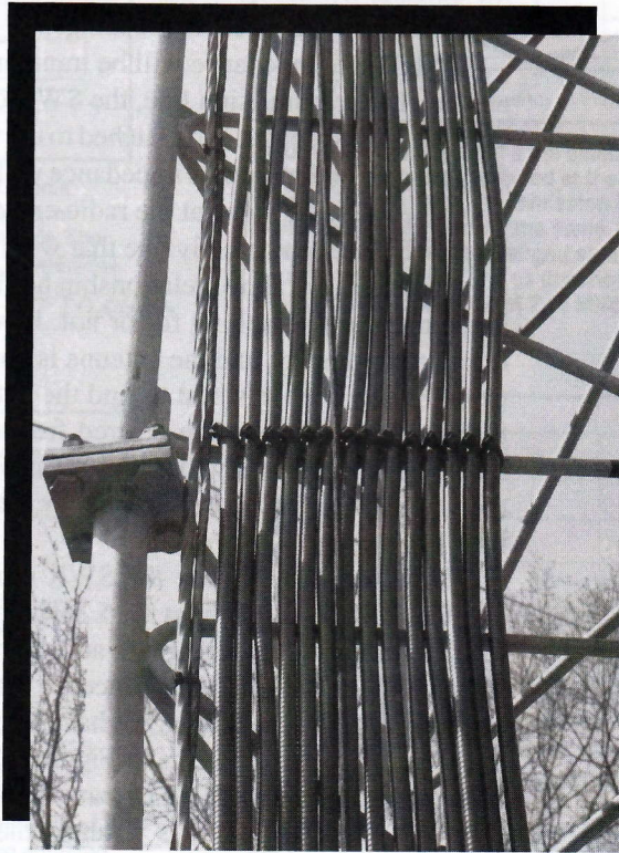
Coaxial cables going up one of the towers at W1AW, the ARRL Headquarters station.
