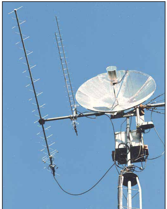
Fig 23.70—The completed and tower-mounted AO-40 antenna system ready to go! The 40-W, 23-cm amplifier is enclosed in the box below the dish antenna.
