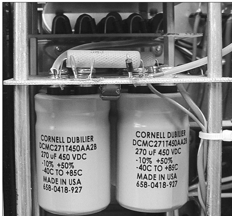
Fig 7.45 — Example of the filter capacitor/bleeder resistor installation in a high voltage power supply.
