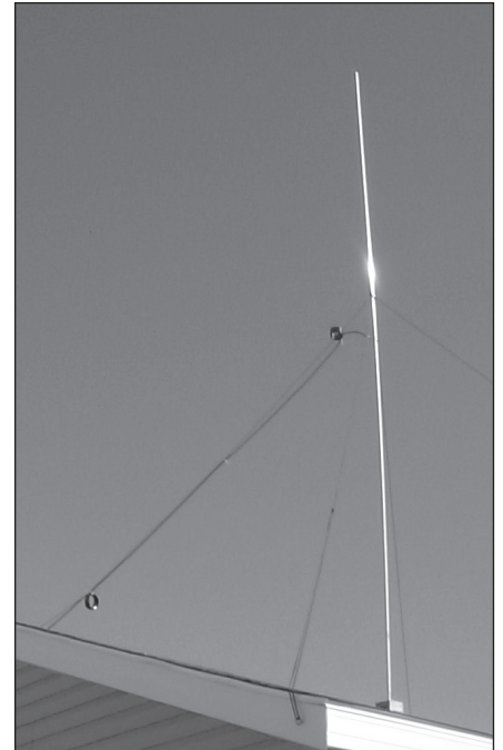
Fig 21.65 — The HVD installed at K8CH. An eye screw that is used for securing one of the guy lines is visible in the foreground. You can also see the two choke baluns that are used in the feed system (see text).
