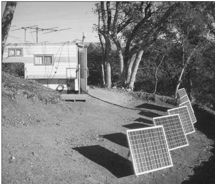
Fig 29.30 — Solar panels can be used to charge a bank of batteries to supply power. Effective off-grid power requires an accurate and conservative estimate of power needs and available energy sources. (K6VVA photo)
