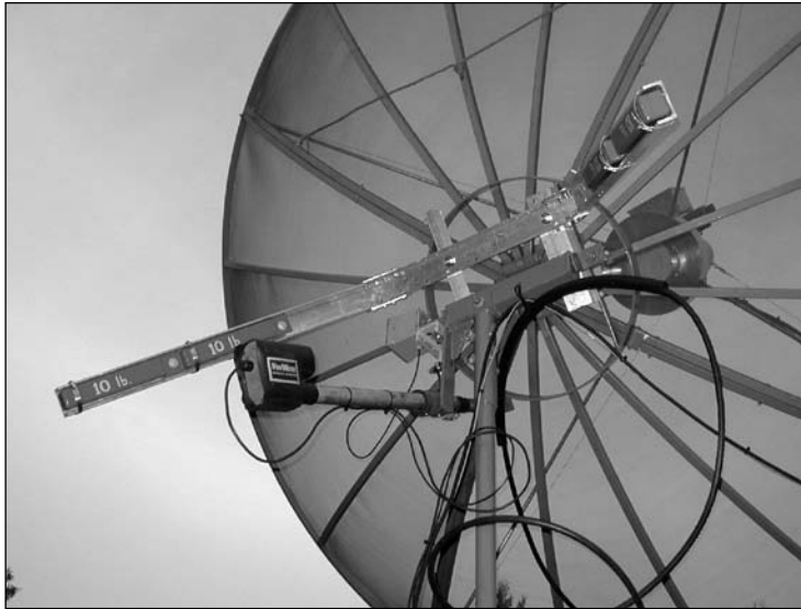
Fig 71 — Mounting arrangement, counterweights and az/el control system for the VA7MM 3 m dish.
