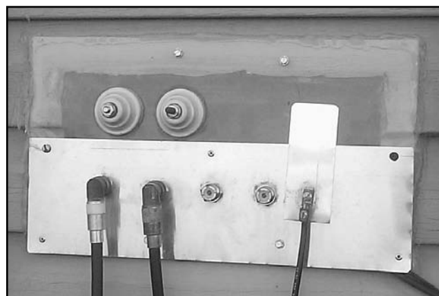
Fig 45 —K8CH's coax entry panel mounted on exterior wall (later covered by grill that provides combustion to an unused fireplace). The ground braid goes to a ground rod located beneath the panel. (Photo courtesy: Simple and Fun Antennas for Hams )
