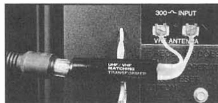
Figure 6.8—This is how to use 75- \Omega coax with a 300- \Omega TV antenna and television.
