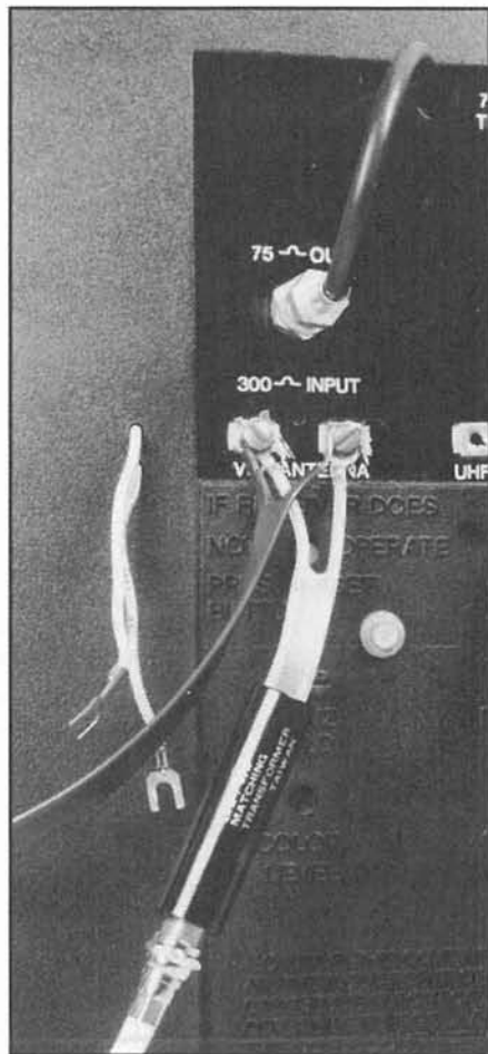
Figure 7.4—The 300- \Omega twin lead used in this illegal CATV hookup certainly causes CATV leaks and results in interference to and from amateur stations. All CATV installation work should be done by CATV personnel.
