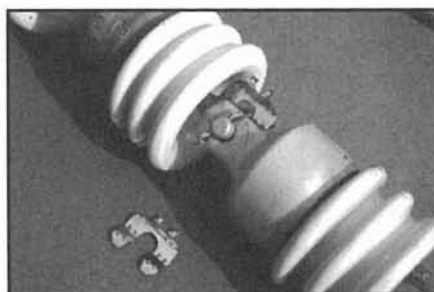
Figure 11.18—These "bell" insulators are rarely the direct cause of RFI noise. If the line that is connected to them is too slack, however, the internal components can corrode and arc.
