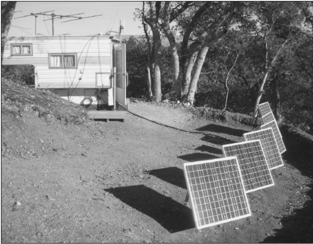
Figure 24.49 — Solar panels can be used to charge a bank of batteries to supply power. Effective off-grid power requires an accurate and conservative estimate of power needs and available energy sources. [Rick Hilding, K6VVA, photo]
