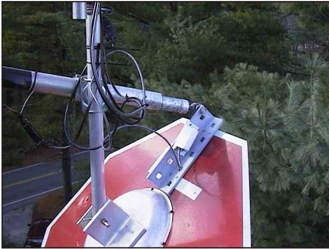
Fig 3 —A rear view of the flyswatter assembly with the tilt sensor in place (white box on the angle bar). The swivel caster that permits the actuator to swivel is mounted near the top of the mast, among several cables. As the actuator lengthens or shortens, it adjusts the angle of the flyswatter to alter the takeoff angle of the antenna beam. A rotator at the top of the mast moves the flyswatter to set the azimuth of the antenna beam.
