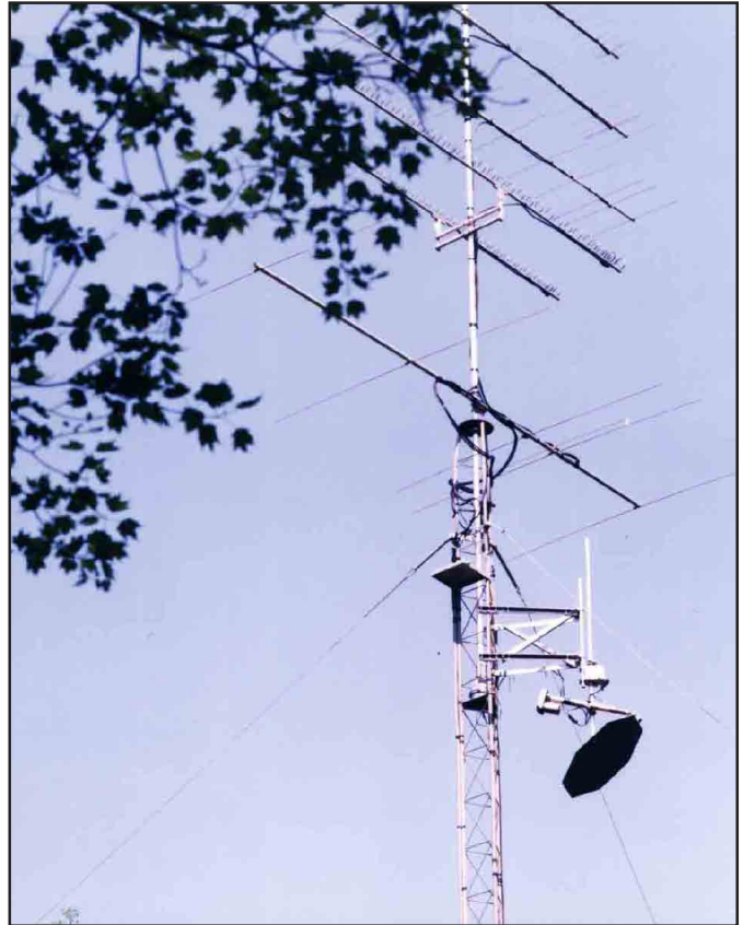
Fig 6 —The complete flyswatter assembly mounted at the top of a tower.
