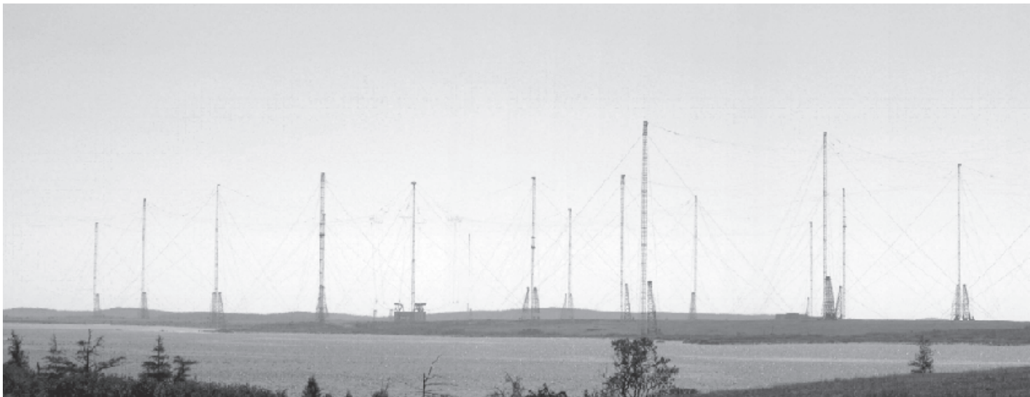
Figure 8 — Here is a photo of the antenna field for station NAA in Cutler, Maine.
