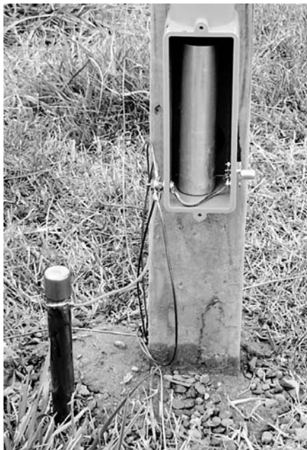
Figure 19 — You can see the ground rod and radial attachment for a vertical in this photo.
