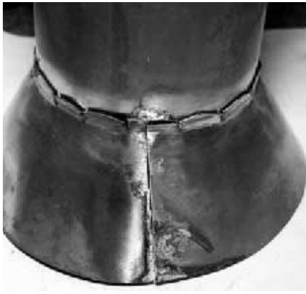
Figure 16 — Cylinder with flange fitted over pipe ready to solder. This may take quite a bit of heat.
