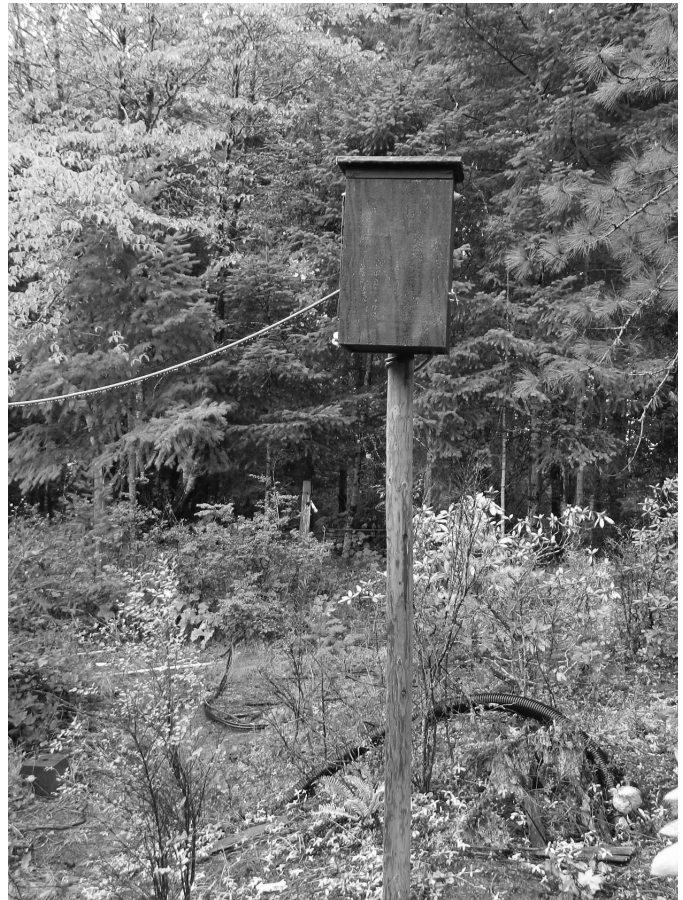
Photo F — The driven element's east leg tuning box. The heavy cable contains the low-voltage control wires.
