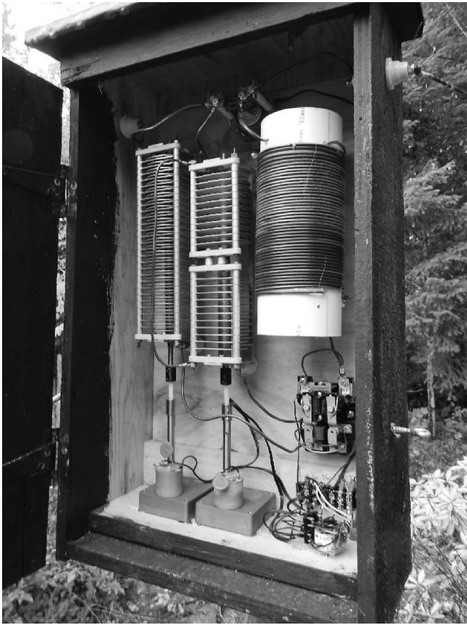
Photo G — Inside the east leg box: The high voltage switch at the top inside the box shorts the inductor out for broadside patterns. The lower voltage switch selects one of the two variable capacitors. These capacitors are in series with the fixed inductor, which is wound on a PCV pipe section. These capacitors are connected in series with the inductor and provide motor-driven variable tuning for the east and west end-fire patterns. The small relay at the bottom automatically connects the appropriate motor/capacitor for either the east or west pattern. These capacitors must be mounted on insulators. Notice also the nylon insulators connecting to the motors. The motors are 12 V DC, 6 rpm gear motors. The DC control permits easy direction changing when fine tuning the antenna.
