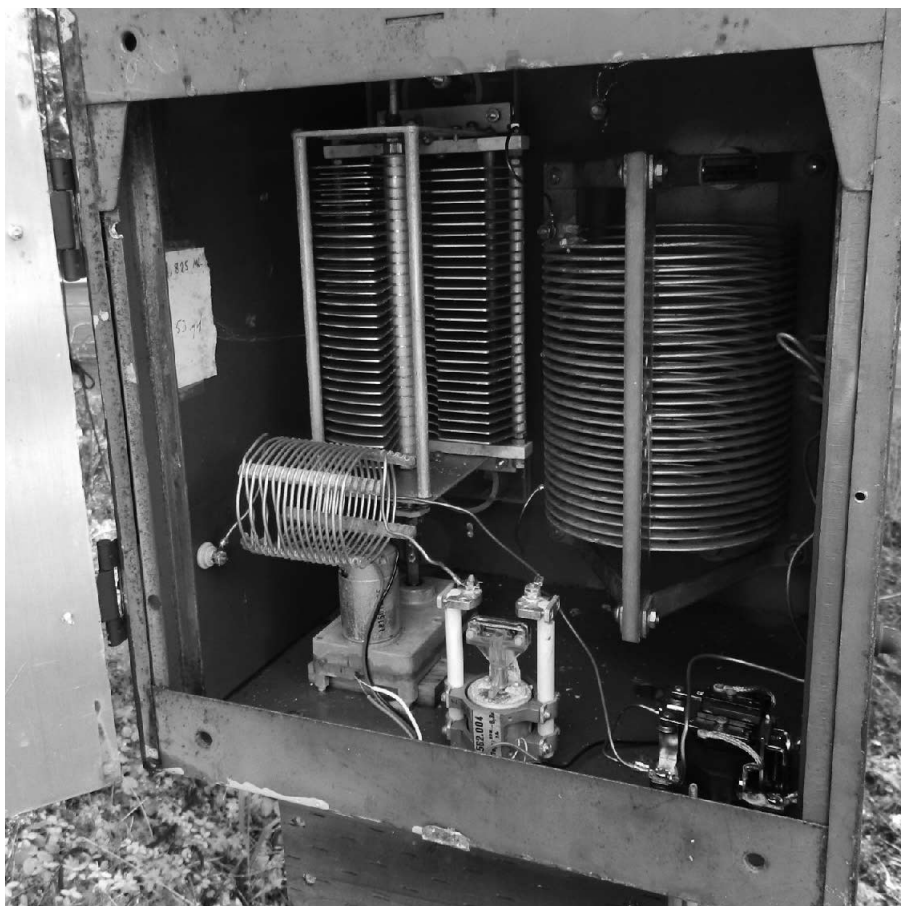
Photo 1 — This is a peek inside the parasitic loop tuning box. The high voltage surplus Russian switch is used to close the loop, thus activating the loop. A remote controlled motor-driven variable capacitor is used in series with the inductor to provide a continuously variable inductance. Thus the array can be adjusted from the shack for maximum forward gain or maximum F/B. A second lower-voltage switch is used to tap the inductor for a director pattern toward New Zealand. The director pattern is a “free feature” but is not very critical, thus fine tuning is not required. The box is an old single-drawer file cabinet with an aluminum sheet access door. The exterior of the box was painted with rust-resistance paint.
