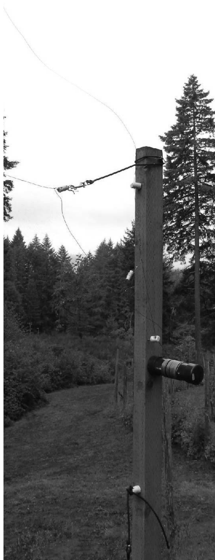
Photo J — Here is the west corner of the parasitic loop: A fixed inductor wound on a 3 inch ABS plastic pipe section with insulated #12 electrical wire solves the problem. ABS end connectors are used to close the pipe and provide a convenient mounting scheme on the post. Note the west anchor for the horizontal wire at the top of the pole using a bungee cord for stress relief. The vertical wire is fed through a ceramic electric fence insulator near the top of the post and with stress relief provided by another bungee cord. My pinot noir vineyard is in the background.
