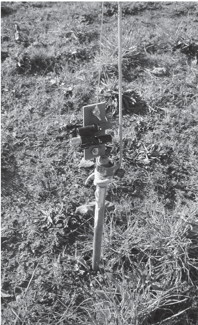
Figure 29 — Feed point and ground rod of test antenna #3.
