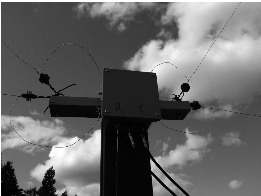
Figure 23 — Transformer box at the center of the array.
