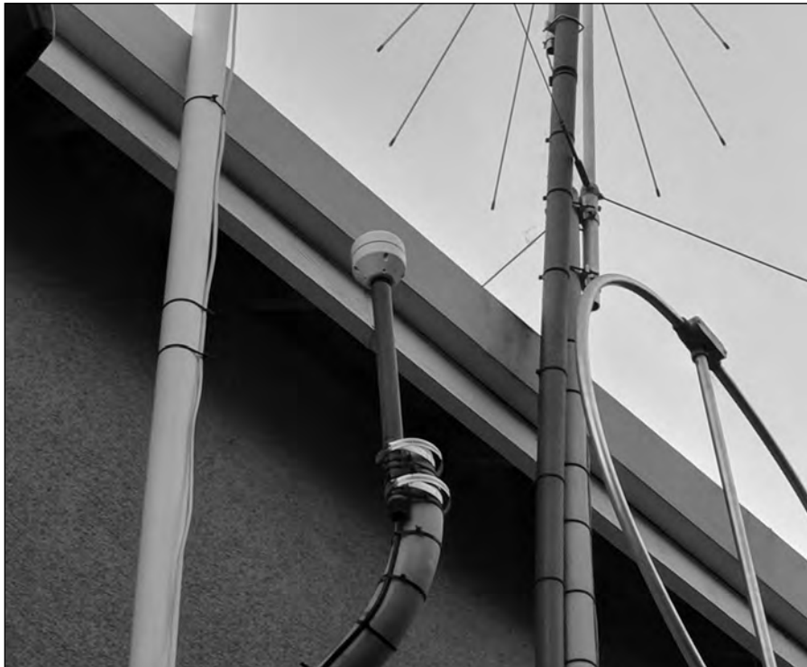
Figure 14 — GPS timing antenna.
