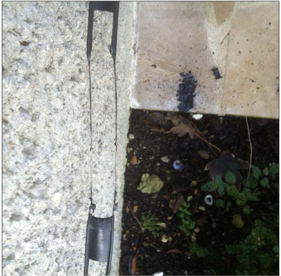
Figure C — Burned-out insulation of the window transmission line section.
