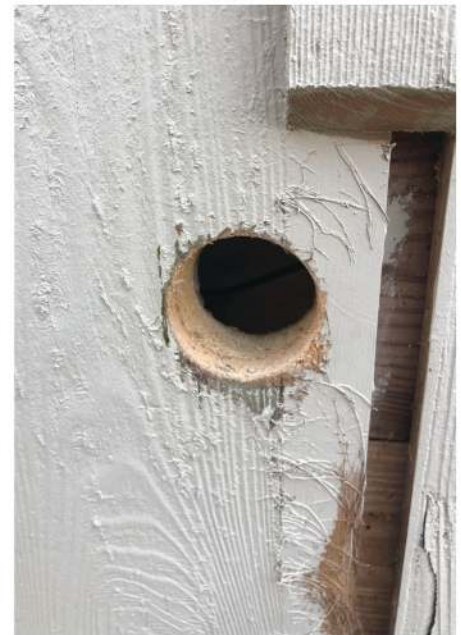
Photo 5 — 2+ inch hole for conduit.
