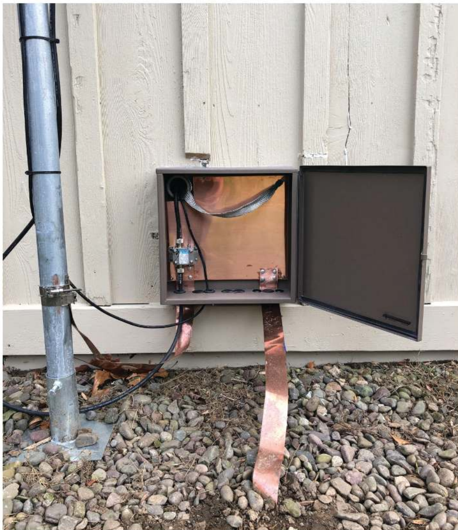
Photo 6 — Entrance panel box with coax lightning arrestor, ethernet from UBB to switch and tinned copper braid from station ground bar.
