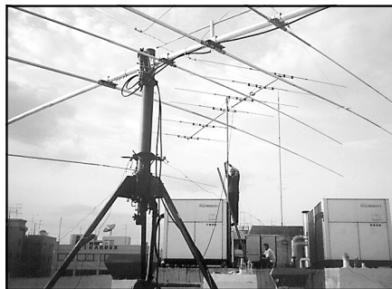
The antenna farm on the roof of the hotel. The Force 12 C4SXL is in the foreground and the PKW 6-element 10-meter Yagi is in the background. Perhaps we should try to negotiate with Force 12 for some sponsorship in exchange for attempting to secure C4SXL as a contest call sign?
