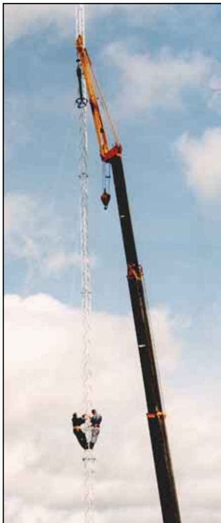
A crane lifting the 140-foot rotating tower with OH1EH and OH1JT along for the ride.
