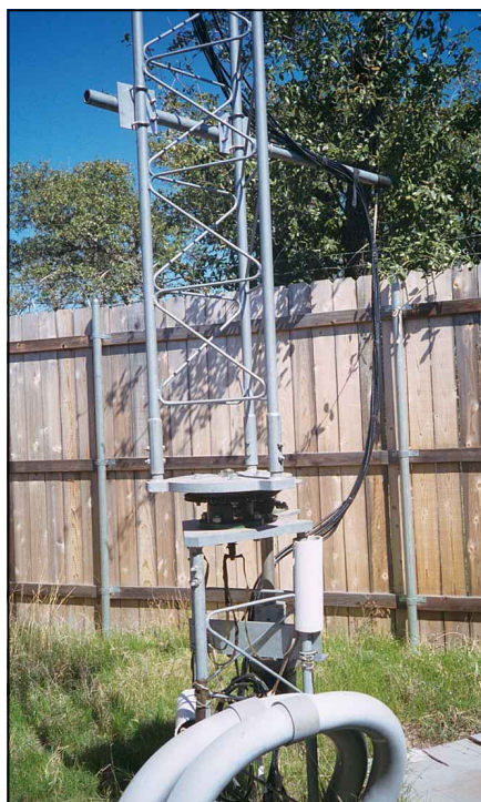
A close-up of the rotor mechanism on the 195-foot rotating tower at N5CQ.
