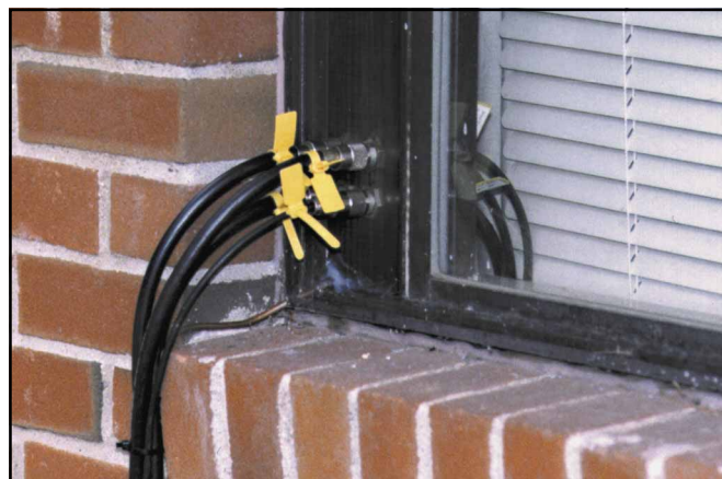
My improvised “window treatment” passes several coaxial feed lines and my ground wire.
