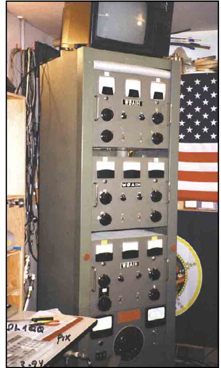
Paul built several of these W0IH-designed 4-1000 amps 35 years ago. They're still running strong. (Photo by DL1QQ)
