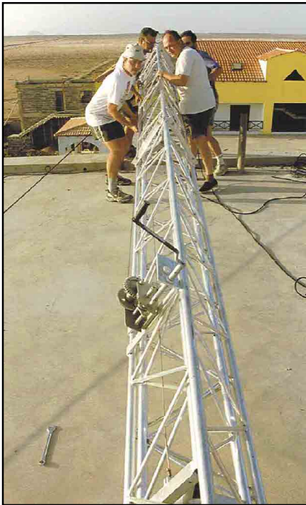
The second tower is being raised. On the left are Gabriele, IK4UPB and Xara, CT1EKF. On the right are Fabio, I4UFH and Vittorio, I4YSS.
