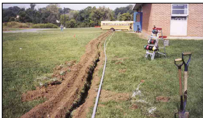
All great tower installations feature a trench, and Hermann Bearcat ARC members took shovels and trenching machine in hand for this schoolyard effort.
