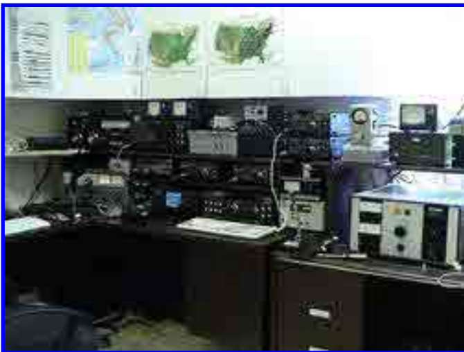
6Meters= ICOM756Pro + VHF-1200; 2Meters = IC-275H + Henry 2002A; 222 = TS2000X + DEMI transverter + TE Systems 300w Amp; 432Mhz = IC-475A + D1010; 903Mhz = IC-275A + DEMI Transverter; 1296Mhz = TS2000X; 2304Mhz = TS2000X + DEMI Transverter + 10 watt amp
