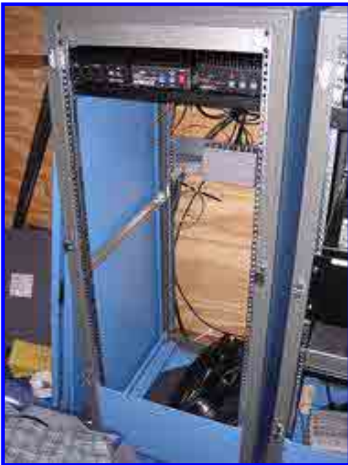
The VHF Amp Rack (Lots of room for more power!)
