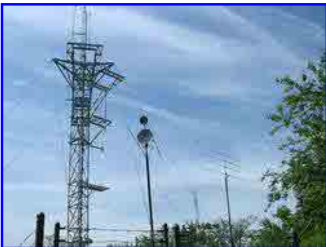
VHF & Microwave Towers
