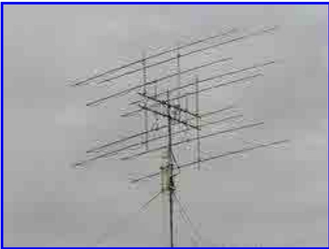
2 meter beam center top, 222 outside 4 antennas, 432 inside 4 antennas
