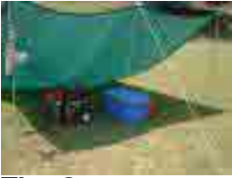
The Generator and noise abatement system (a tarp)!
