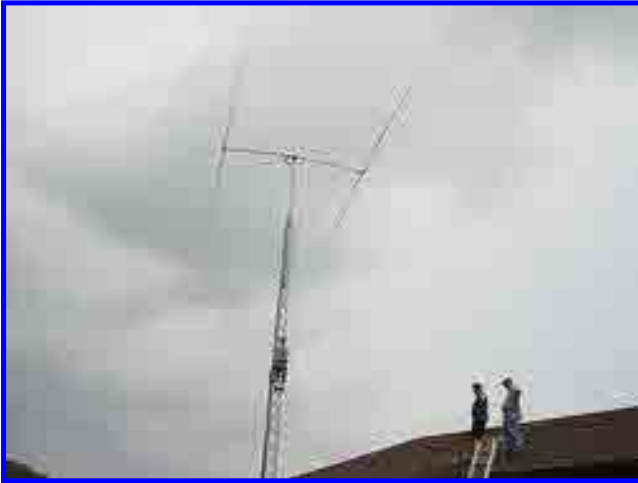
The big tower with the 40m 2 element beam just after being raised, it took a big chunk of effort to get this one up !
