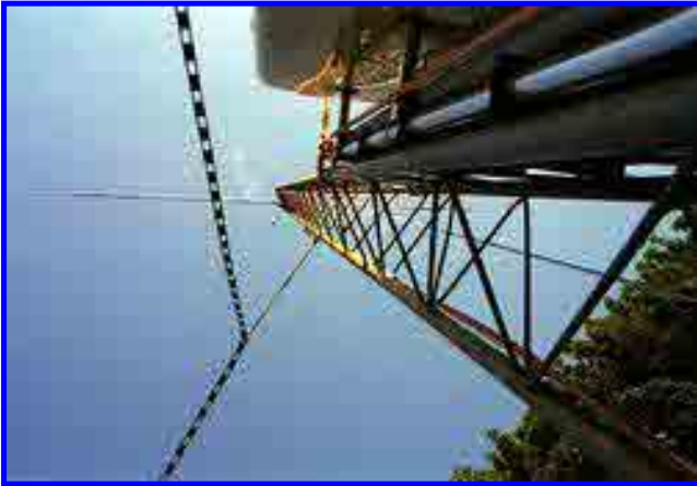
The tower is up! A triband rotatable dipole and an 80 meter dipole are installed too.
