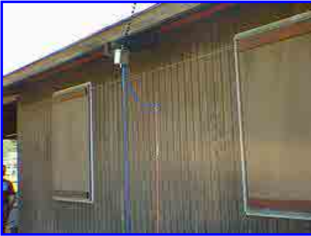
The 9:1 RF Transformer under the pavillion eave showing the 450 ohm ladder line to coax with ground rod.
