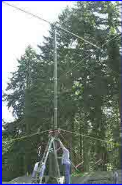
The W7DK tower crew puts the finishing touches on one of the 20 meter Yagis. The Yagis are held up in the air with Army Surplus Crank Up towers.
