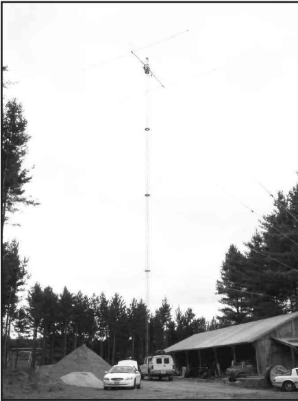
Figure 3—Bolting the Force 12 80 meter Yagi in place at 170' on a Rotating Tower Systems rotating Rohn 55 tower
