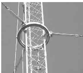
Guy ring bearing installed on Rohn 55G tower.
