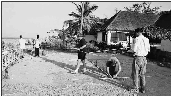
Figure 1—Assembling the 40 meter vertical. From left in the foreground: John, AB6BH, Art, W6XD, (kneeling) and Dick, N6AA.
