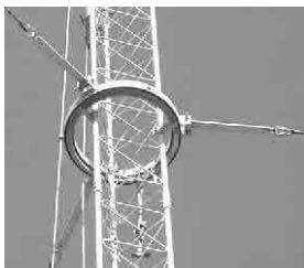
Guy ring bearing installed on Rohn 55G tower.
