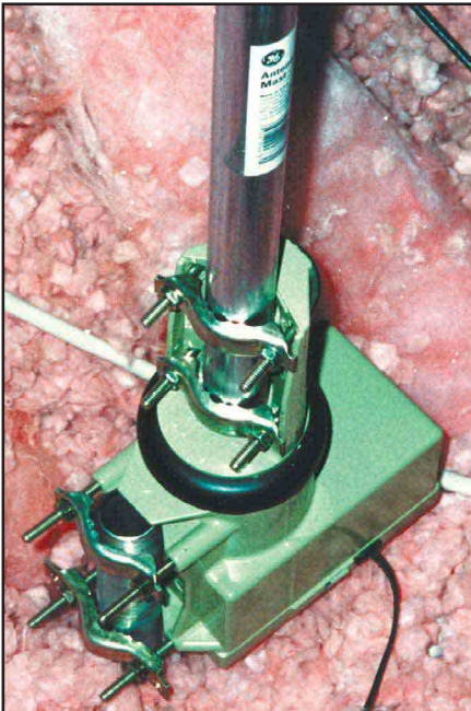
Figure 2—The rotator is mounted to a pipe support secured to a floor member. Ceiling insulation covers the support.
