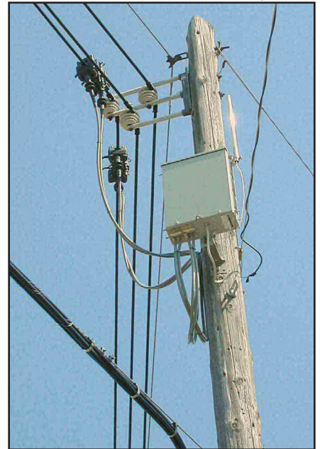
A BPL connection and box at a field trial in Cedar Rapids, Iowa.
