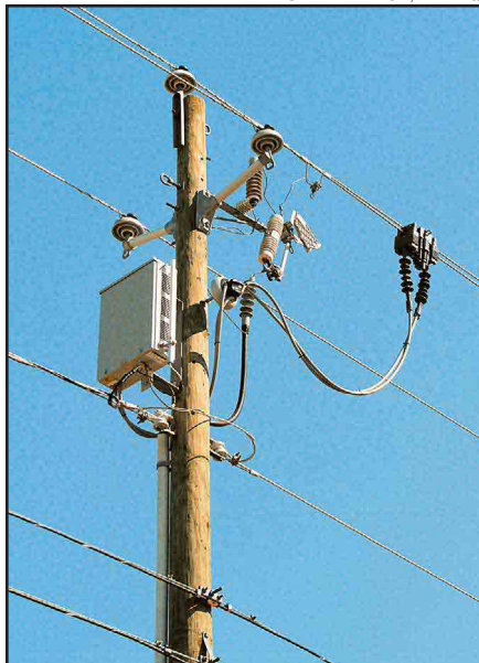
A BPL "extractor" on a Progress Energy pole near Raleigh, North Carolina.
