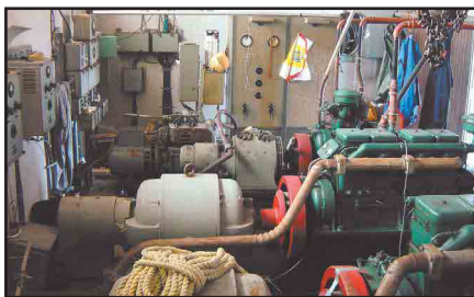
The third building is full of weary generators from the old days. Only a recent 10 kW affair at the far back is powering visiting DXpeditioners.
