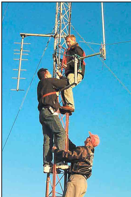
From the top: Dave Warwick, K4DJW; KG4MSU, and John Jaskolka, KR4ZJ, install the 2 meter antenna at Craven Regional Medical Center.
