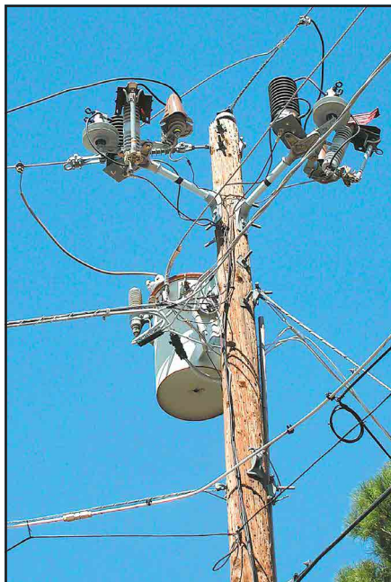
The Cottonwood BPL field trial uses Mitsubishi Electric PLCLINK equipment.
