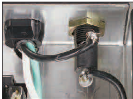
Figure 5 — The MFJ-1164's power cord hot lead is connected to the fuse holder ring terminal, placing 120 V ac near the outside of the cabinet. Reversing the connection so that the power cord hot lead is at the end terminal removes this potential shock hazard.
