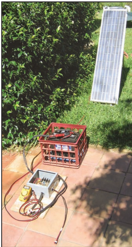
Charging the deep cycle battery with the solar panel. The power distribution assembly (PDA) regulates the charge. The unconnected pigtail is the 12 V dc output from the battery.
