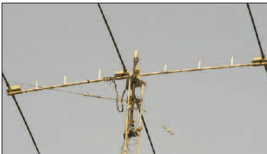
Figure 1 — Yagi with the dipole 8 inches above the boom on six white standoff insulators. The PVC balun and loading coil enclosure is at the top of the mast.
