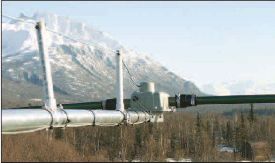
Figure 2 — PVC standoff insulators on boom.
