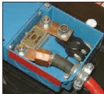
Figure 4 — Battery positive terminal. The 200 A fuse is on left. The link from battery terminal to fuse is made from a 2½ inch length of flattened ½ inch copper water pipe.
