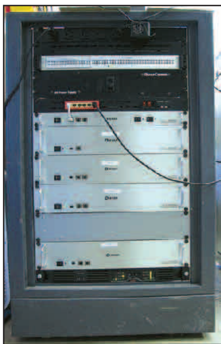
Figure 2 — The full stack of D-STAR equipment at the test bench of Jim McClellan, N5MIJ. From top to bottom, an IP-RP2C controller, an ID-RP2D 1.2 GHz data repeater, an ID-RP2V 1.2 GHz voice repeater, an ID-RP4000 440 MHz voice and data repeater, a blank panel and an ID-RP2000 146 MHz voice and data repeater.
