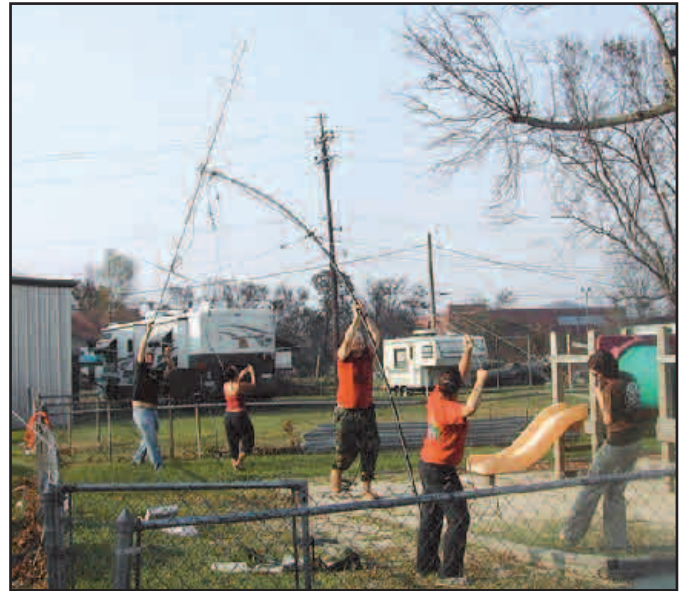
A team of Katrina volunteers from Rhode Island installs a temporary antenna.
